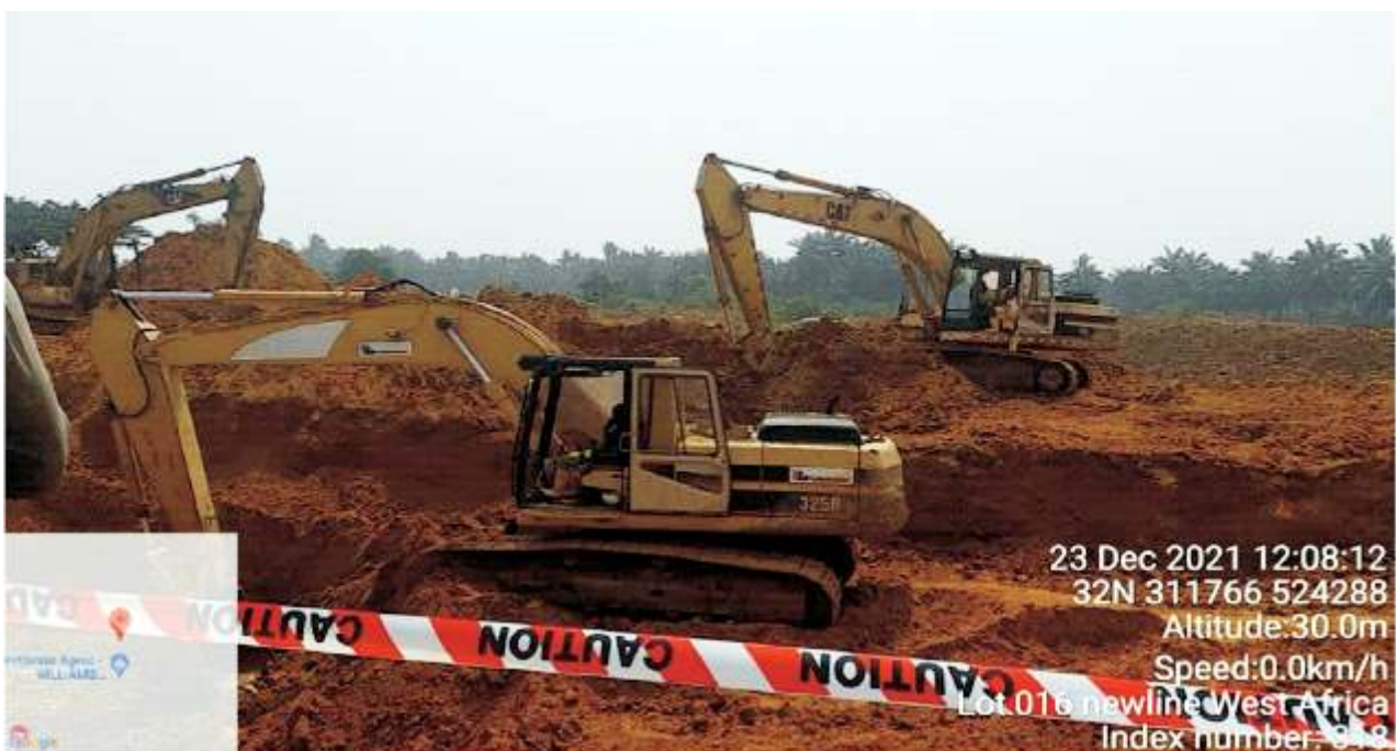
Plate 1.1: Excavation of impacted soil in progress at Lot 016, Buemene Korokoro Well 05, Tai L.G.A. (Contractor: NEWLINE WEST AFRICA LTD)
