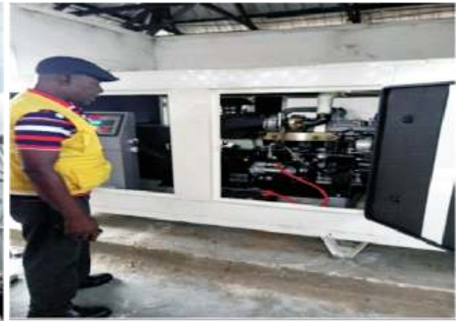
Installed 80KVA Generator at Agbonchia
