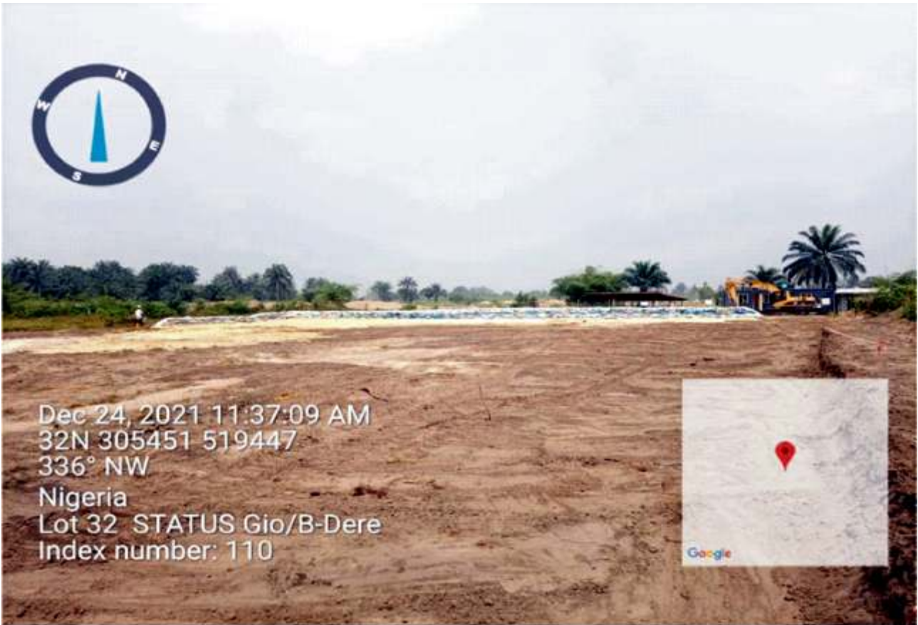
Plate 1.3: Construction of engineered biocell in progress at Lot 032 B.Dere / Gio, Gokana / Tai L.G.A. Remediation Contractor - MOSITO ENVIRON CONSTRUCT LTD
