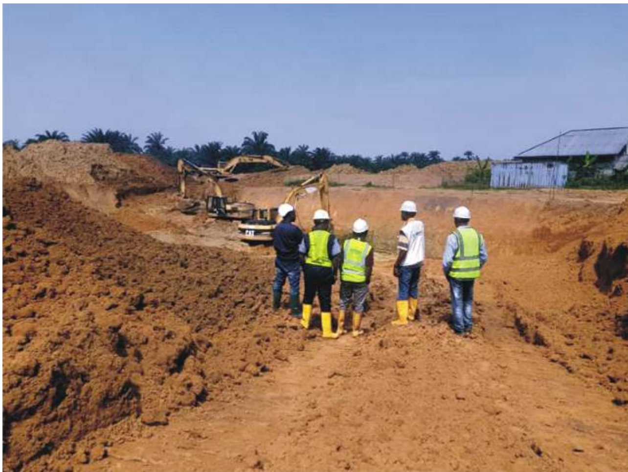
Plate 1.2: Remediation Site Supervisors from HYPREP Operations Unit and Contractor's Site Personnel examining the on-going excavation works at Lot 016, Buemene Korokoro Well 05, Tai L.G.A. (Contractor: NEWLINE WEST AFRICA LTD)
