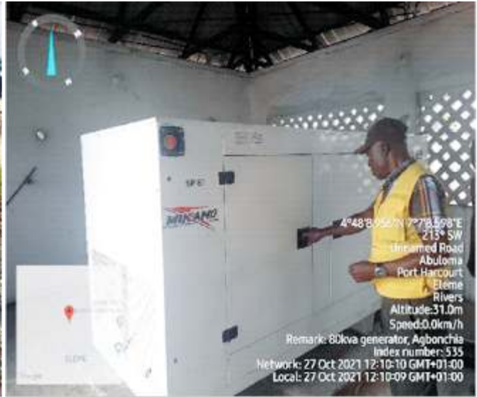
Installed 80KVA Generator at Alesa
