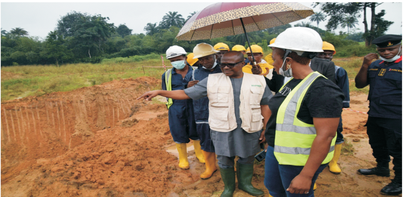
Plate 1.9: The Officer Overseeing the Project Coordination Office (OOPCO) / Head of Operations Unit of HYPREP, Prof. Philip Shekwolo (left) at inspecting work progress at LOT 013 (Nweekol Zorbuke –K.Dere, Gokana L.G.A) with Site Personnel of the Remediation Contractor- Centennial Development and Investments Limited.
