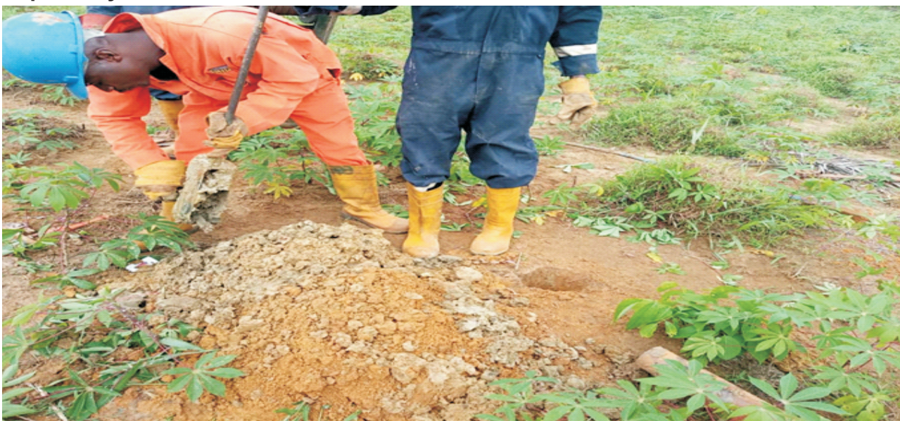
Plate 1.5: Preliminary soil augering preparatory to percussion drilling for installation and development of groundwater monitoring boreholes at Barayiamaa, Kpите, Tai L.G.A for delineation of the site.
