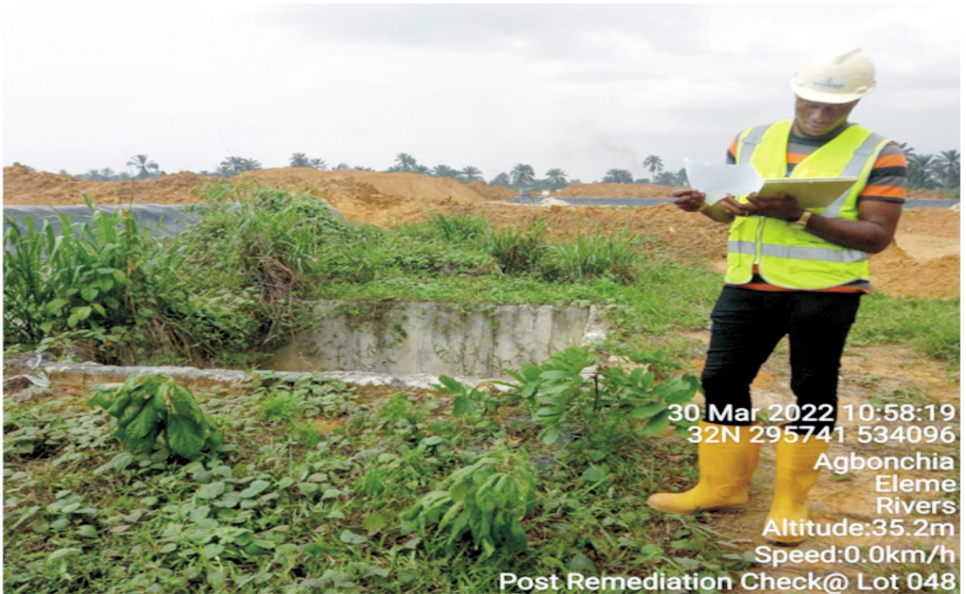
Plate 1.11: Team of Remediation Supervisors undertaking checks on levels of compliance with completion of remediation earthworks and decommissioning of site facilities at Lot 048 (Okuluebu, Ogale, Eleme L.G.A).
