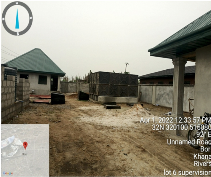
BOOSTER STATION AT A GLANCE
