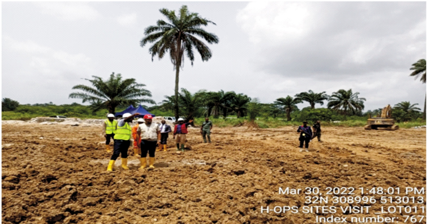
Plate 1.6: Head of HYPREP Operations Unit (in red work jacket) in company of some Sub-Unit Leads examining recently concluded backfilling at Lot 011, Debon, Bodo/Mogho, Gokana L.G.A during one of his routine leadership commitments supervisory sites visits on 30 th March, 2022.
