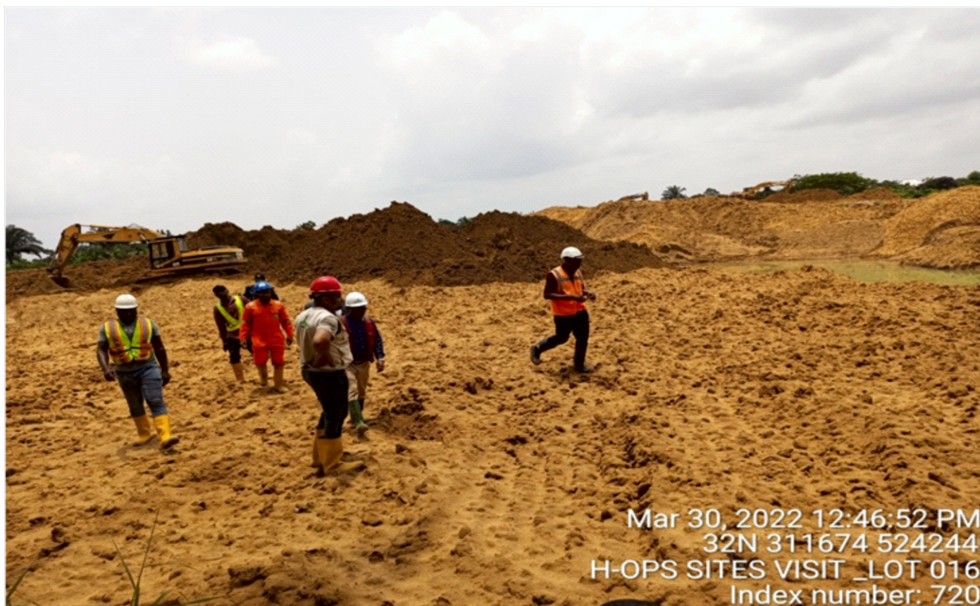
Plate 1.2: On-going backfilling of excavated pits with treated soil at Lot 016, Buemene Korokoro Well 005, Tai L.G.A. (Contractor: NEWLINE WEST AFRICA LTD)
