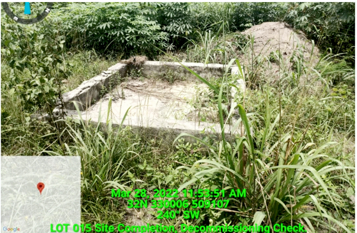
Plate 1.12: Yet to be decommissioned concrete base of the decontamination area at Lot 015 (Wiieborsi -Kpean, Khana L.G.A).
