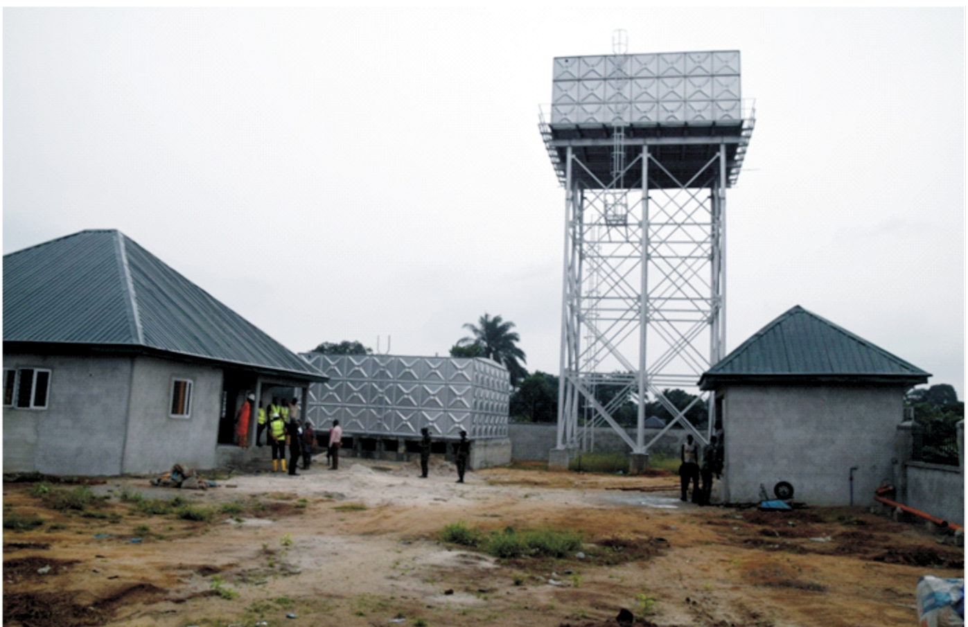
Plate 1.7: Head of Operations visit to HYPREP Potable Water Supply Project under construction at Korokoro, Tai L.G.A during his Supervisory field visit on 3 rd March, 2022.
