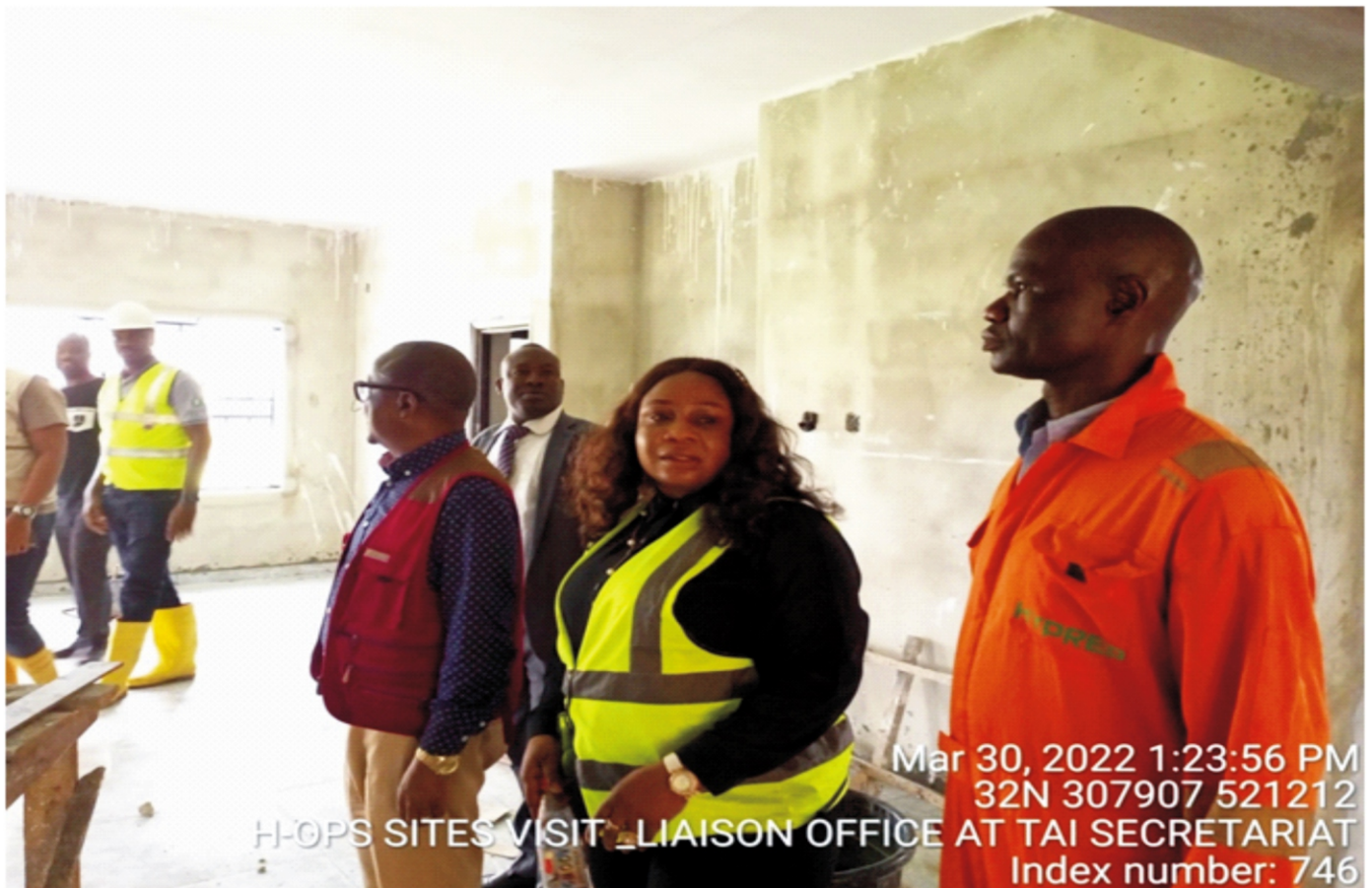
Plate 1.7: Head of Operations visit to HYPREP Liaison Office at Tai Local Government Council Secretariat, Saakpenwa under construction during his Supervisory field visit on 30 th March, 2022.
