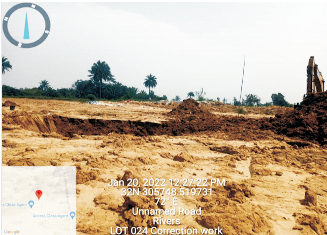
Plate 1.4: Correction of exceedances (retrieval and re-treatment of samples which had higher TPH values than target closure limit from NOSDRA Close-out results) at Lot 024B.Dere / Gio, Gokana / Tai L.G.A. Remediation Contractor-LEVENE ENERGY DEVELOPMENT LTD.
