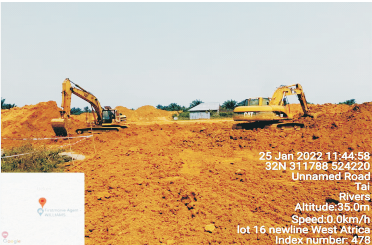
Plate 1.3: Mechanical transferring of excavated impacted soil towards the engineered biocell for treatment on-going at Lot 016, Buemene Korokoro Well 05, Tai L.G.A. (Contractor: NEWLINE WEST AFRICA LTD)
