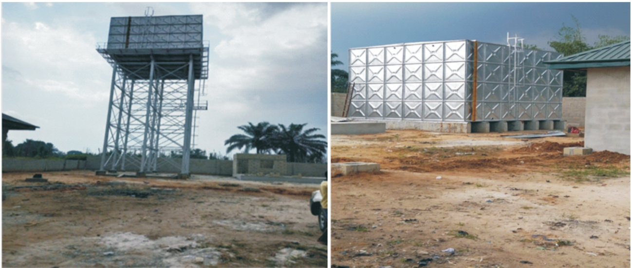
Constructed and installed Overhead and Groundwater Water Tanks at Barako Water Station
