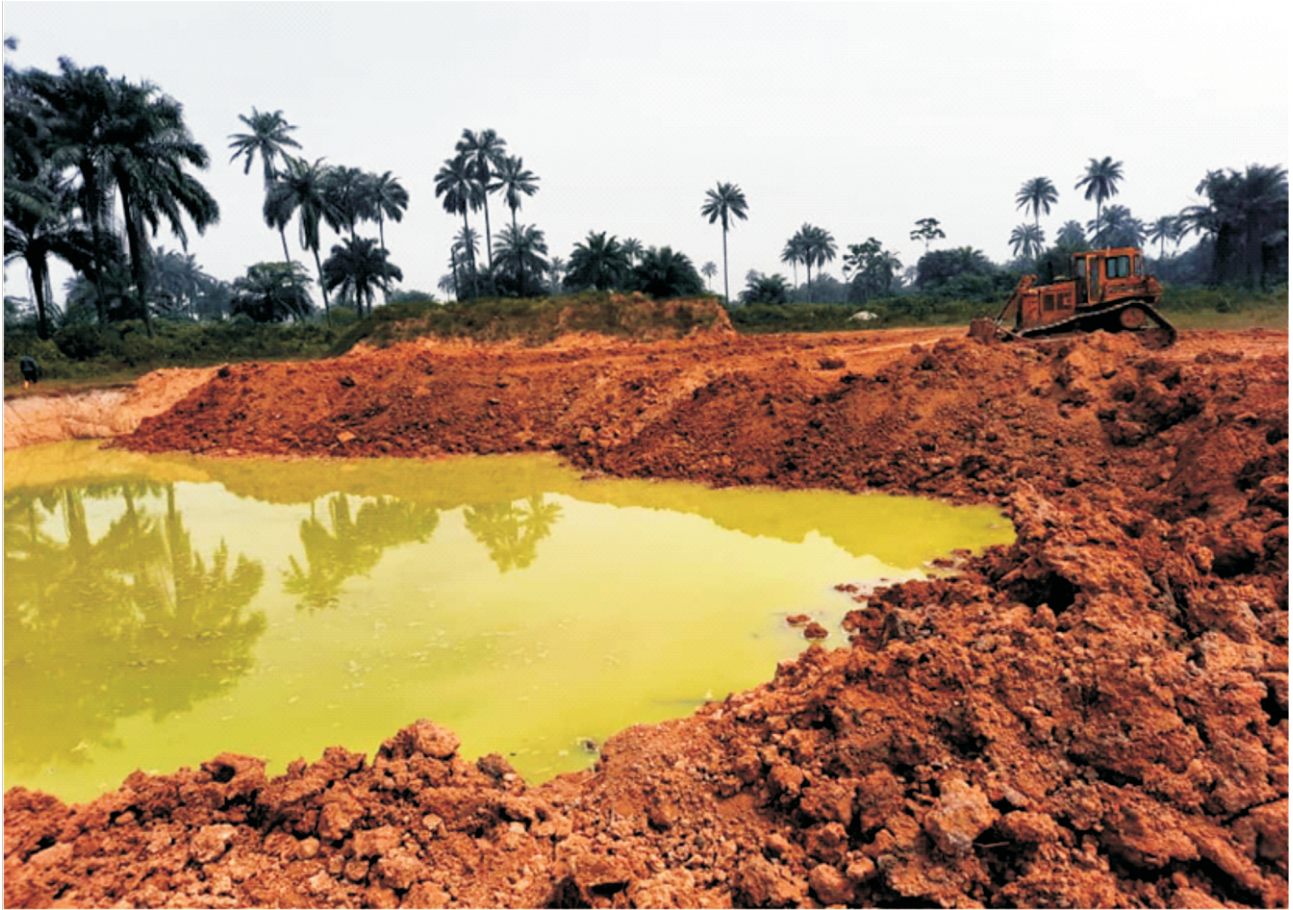
Plate 1.5: Backfilling of excavated pits with treated soil in progress at Lot 046New Elelenwa Manifold, Akpajo, Eleme L.G.A. Remediation Contractor - ANDELSTA LTD.
