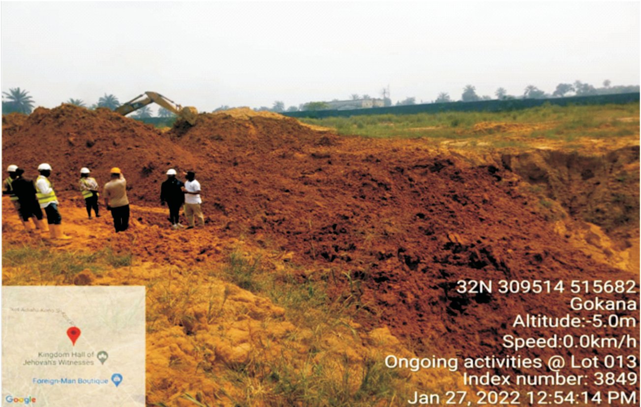
Plate 1.2: HYPREP Operations Unit Remediation Supervisors on routine inspection of on-going backfilling process in progress with Contractor's Site Personnel and Community Workforce Representatives at Lot 013, Nweekol Zorbuke, K.Dere, Gokana L.G.A. (Contractor: CENTENNIAL DEVELOPMENT & INVESTMENT LTD)
