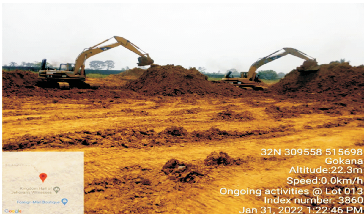
Plate 1.1: Mechanical serial transferring of treated soil from staging area towards the excavated trenches for backfilling in progress at Lot 013, Nweekol Zorbuke, K.Dere, Gokana L.G.A.
