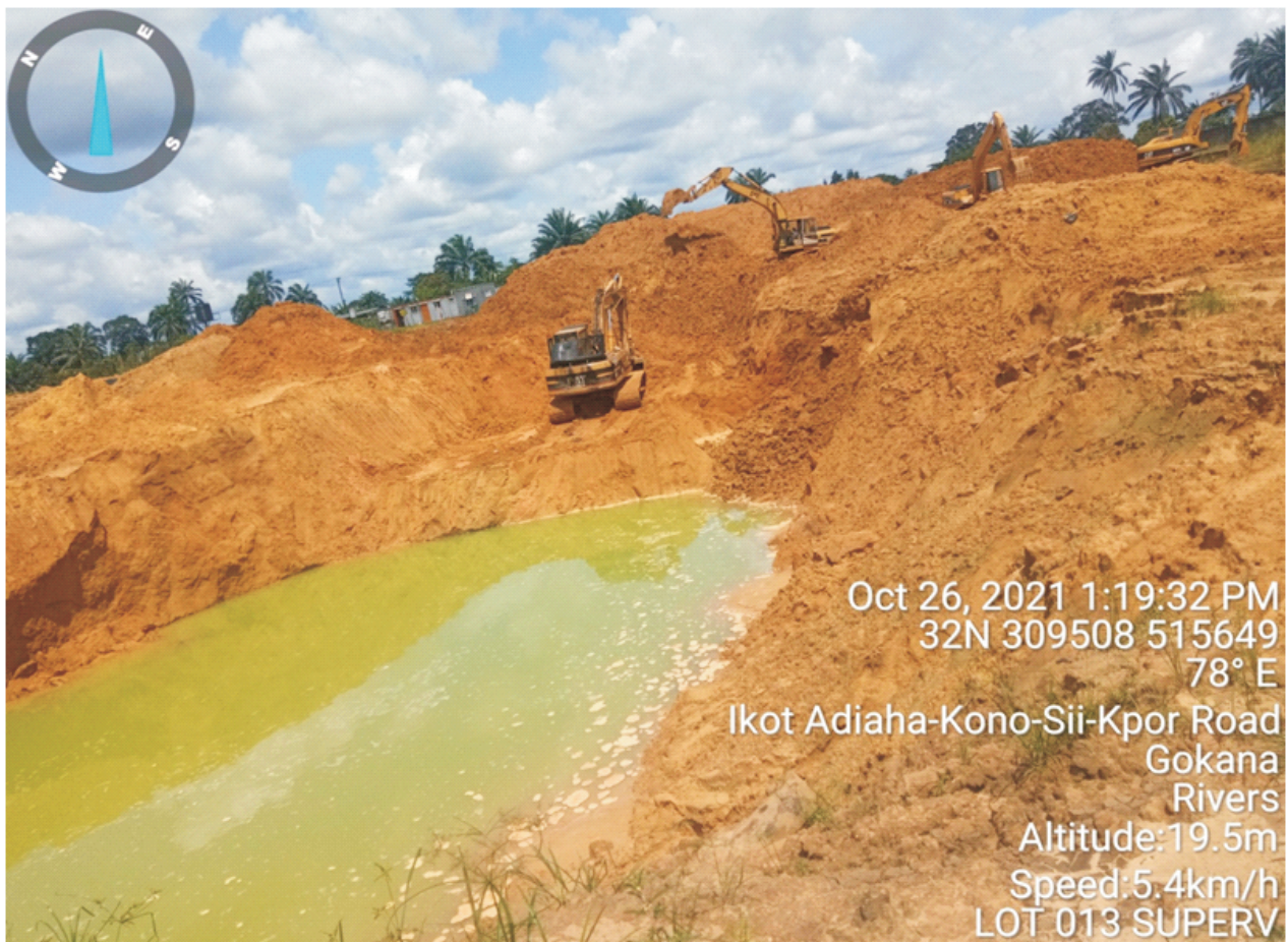
Plate 1.1: Concluding stage of excavation of impacted soil for treatment in progress at Lot 013 (NweekolZorbuke in K. Dere, Gokana L.G.A). (Remediation Contractor - CENTENNIAL DEVELOPMENT & INVESTMENT LTD).
