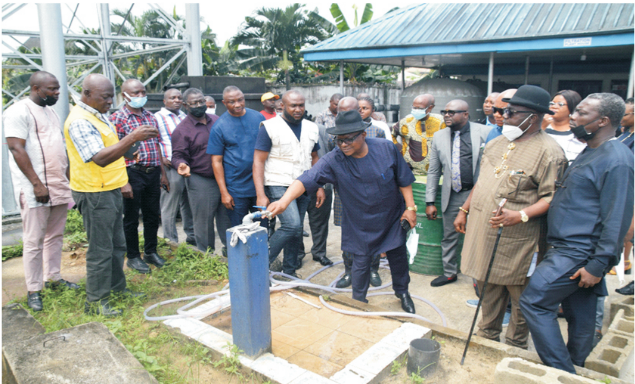
The Project Coordinator, Prof. Philip Shekwolo test-running the Water Supply System at Alesa
