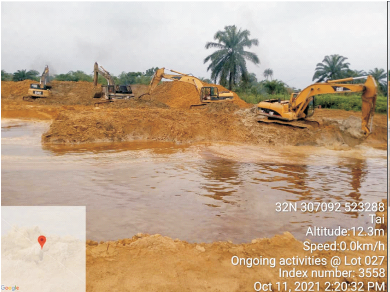
Plate 1.2: on-going excavation and serial transferring of impacted soil in progress at Lot 027 (Bara Alue, Tai L.G.A). Remediation Contractor- EMAMEDNIG. LTD.
