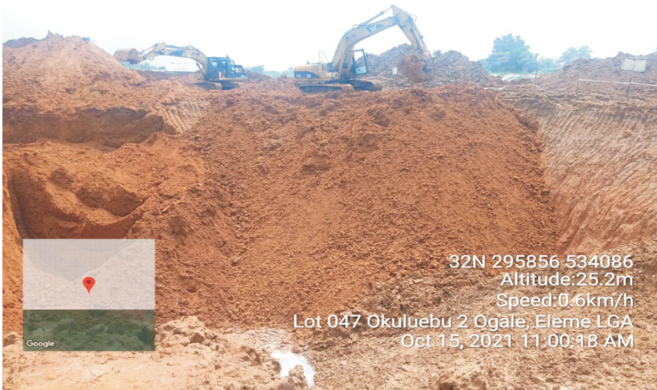
Plate 1.3: Completion of backfilling of excavated pits with treated soil at Lot 047 Okuluebu (Ajeokpori Well 3) –Ogale, Eleme L.G.A. Remediation Contractor - LAPIDEO MULTI SERVICES LTD.
