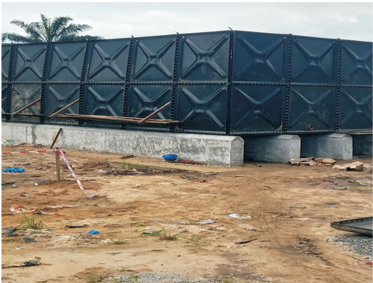
Installed Ground Tank at Barako
