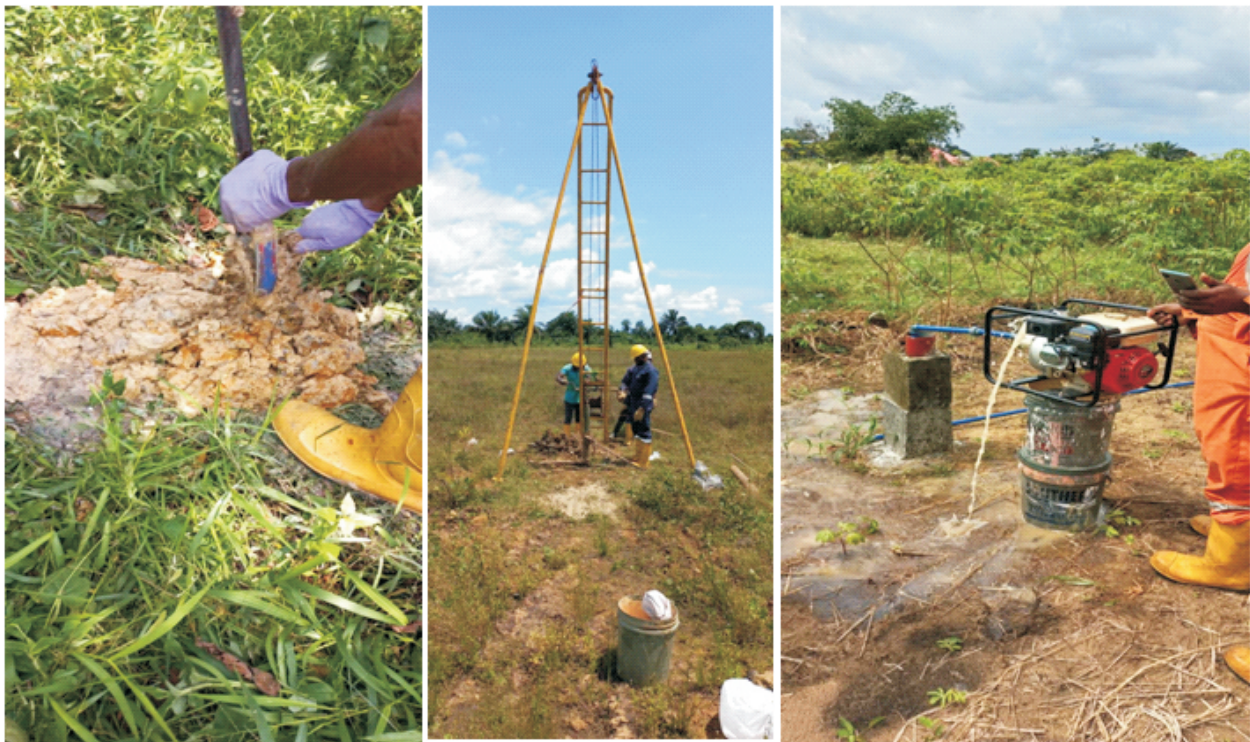
Plate 1.5(a-c): Preliminary soil augering preparatory to percussion drilling, percussion drilling and mechanical flushing of installed groundwater monitoring boreholes at Barabeedom, K. Dere in Gokana L.G.A for delineation of the site.
