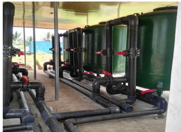
Plate 4.4b: Internal connection of pressure filters at Terabor station.
