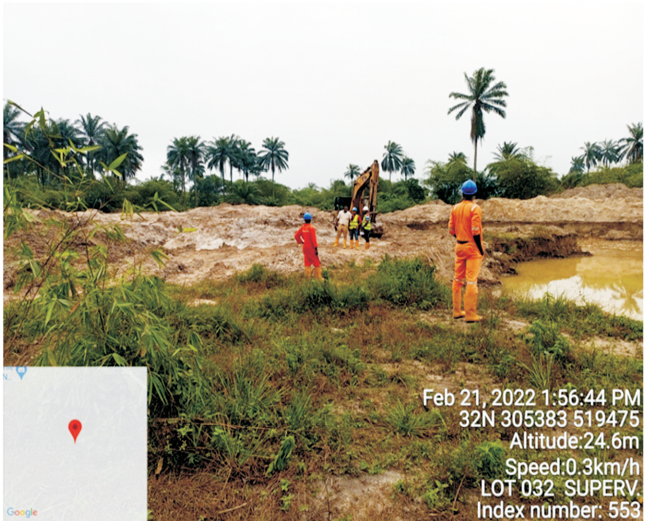
Plate 1.5: Excavation of impacted soil for treatment at Lot 032 in B. Dere / Gio, Gokana / Tai L.G.A. Remediation Contractor - MOSITO ENVIRONMENTAL LTD.
