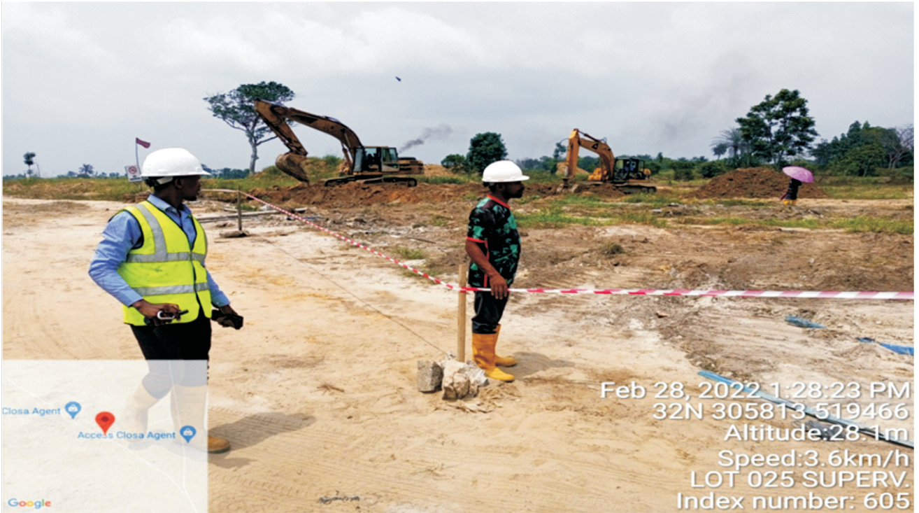
Plate 1.3: Mechanical excavation of the final segment of impacted soil for treatment in progress at Lot 025 B.Dere / Gio, Gokana / Tai L.G.A. Remediation Contractor - SUBADOM GLOBAL RESOURCES LTD.
