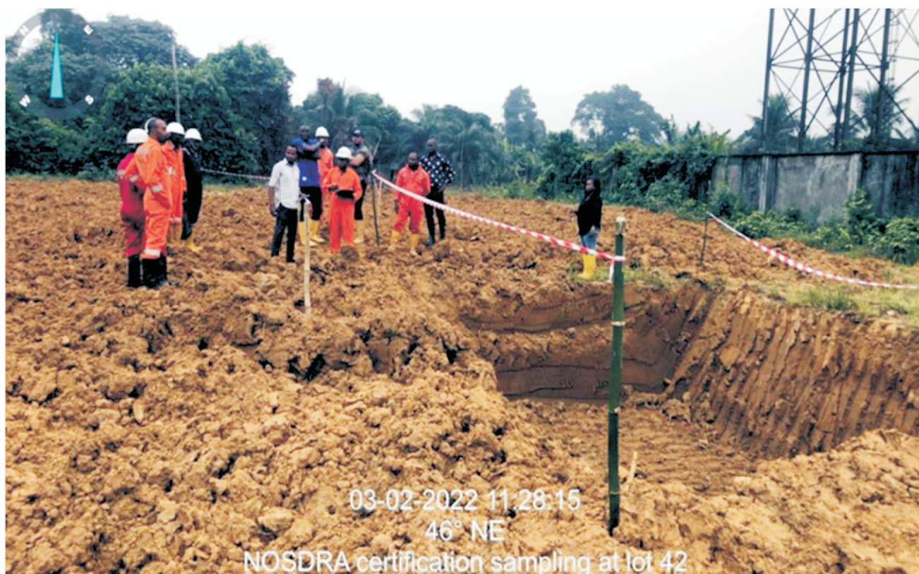
Plate 1.6: NOSDRA re-sampling soil with initial exceedances after re-treatment at Lot 042 Korokoro Well 4, Tai L.G.A. Remediation Contractor: KANNY KOY LTD
