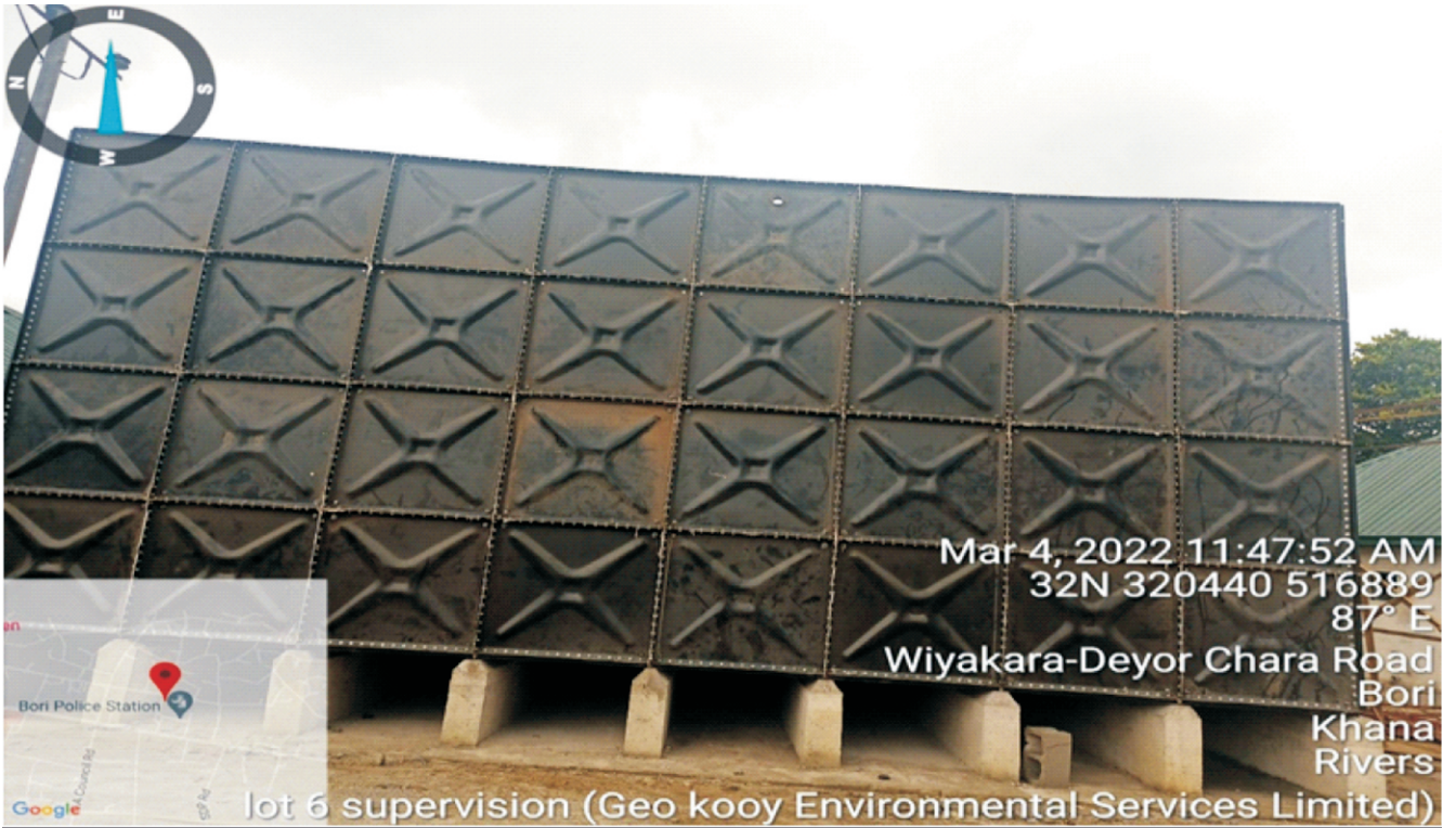
Installed Surface tank at Bori
