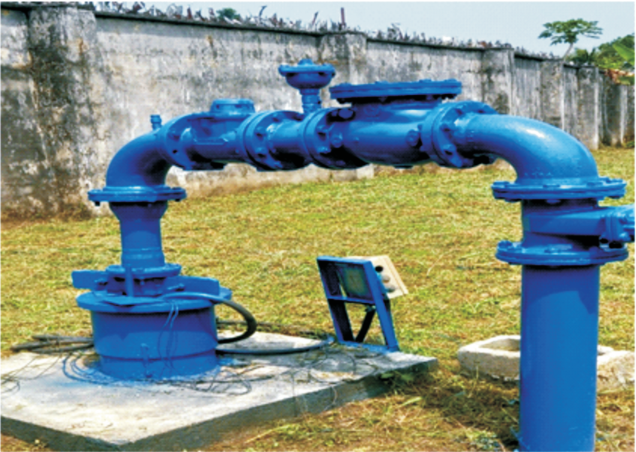
Complete installed Borehole head at Terabo
