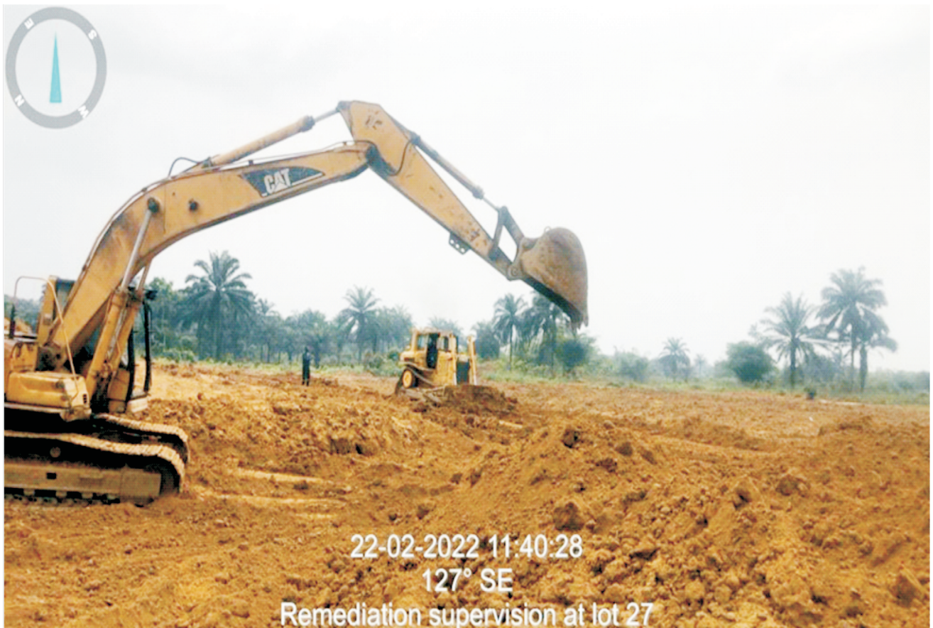
Plate 1.4: Final stage of backfilling, site leveling and landscaping in progress at Lot 027 (Bara Alue, Tai L.G.A). Remediation Contractor - MARM CONSULTING SERVICES LTD.
