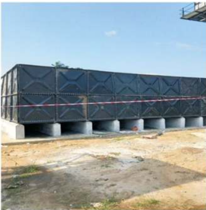
Installed Ground tank at Terrabo
