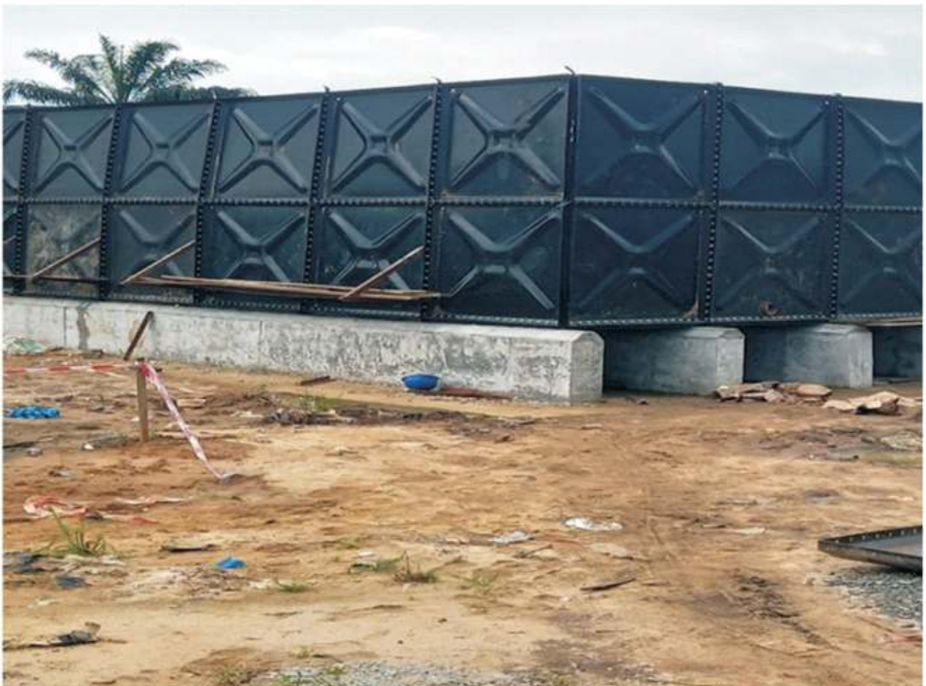
Installed Ground Tank at Barako
