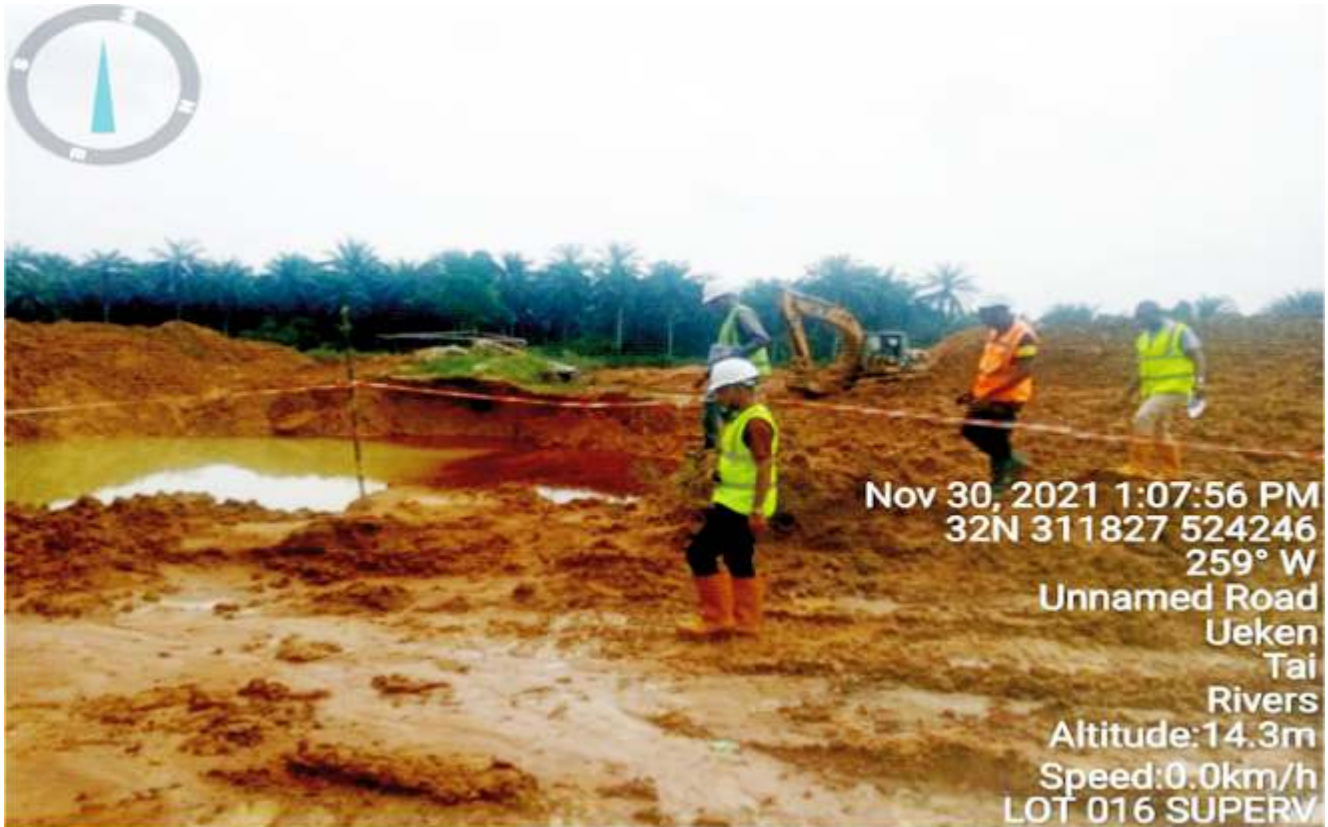
Plate 1.2: Serial transfer of excavated impacted soil in progress at Lot 016, BuemeneKorokoro Well 05, Tai L.G.A.(Contractor: NEWLINE WEST AFRICA LTD)
