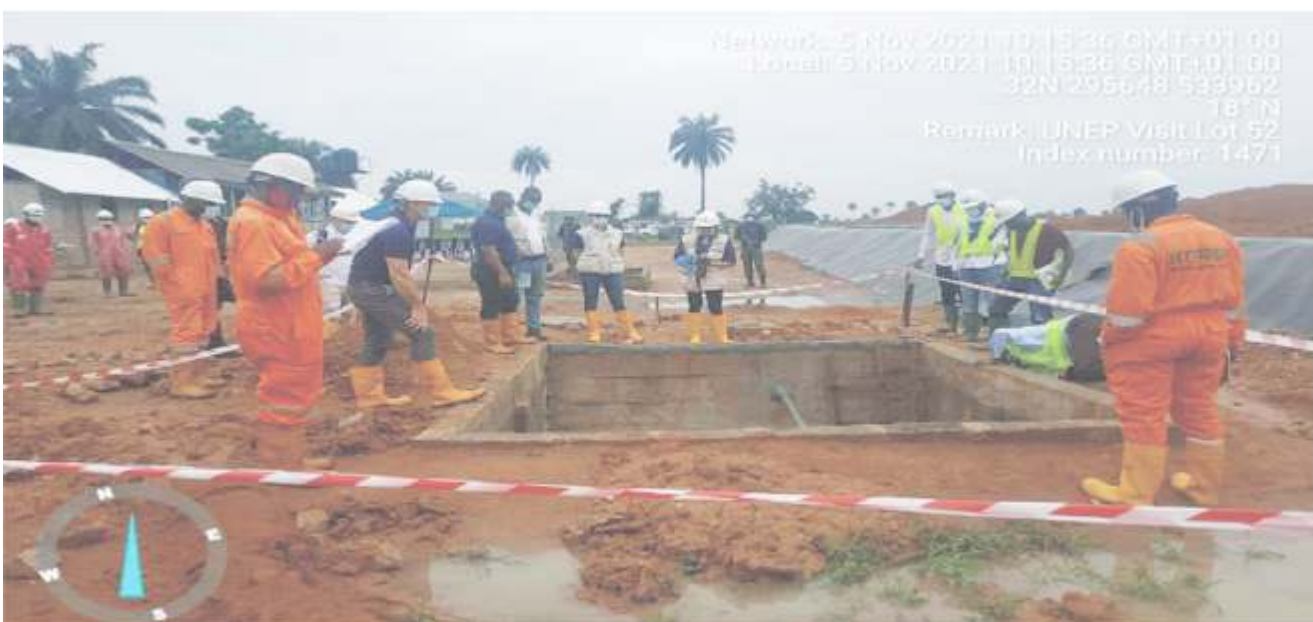
Plate 1.6: The UNEP Joint Team inspecting the leachate sump at Lot 052 at the Okuluebu 2 (Ajeokpori Well 3), Ogale, Eleme L.G.A Remediation Cluster site for Lot 047 – 055.
