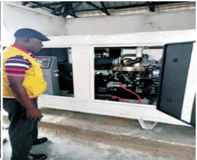
Installed 80KVA Generator at Agbonchia
