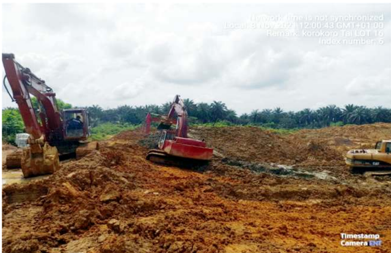
Plate 1.1: Excavation of impacted soil in progress at Lot 016, BuemeneKorokoro Well 05, Tai L.G.A. (Contractor: NEWLINE WEST AFRICA LTD)
