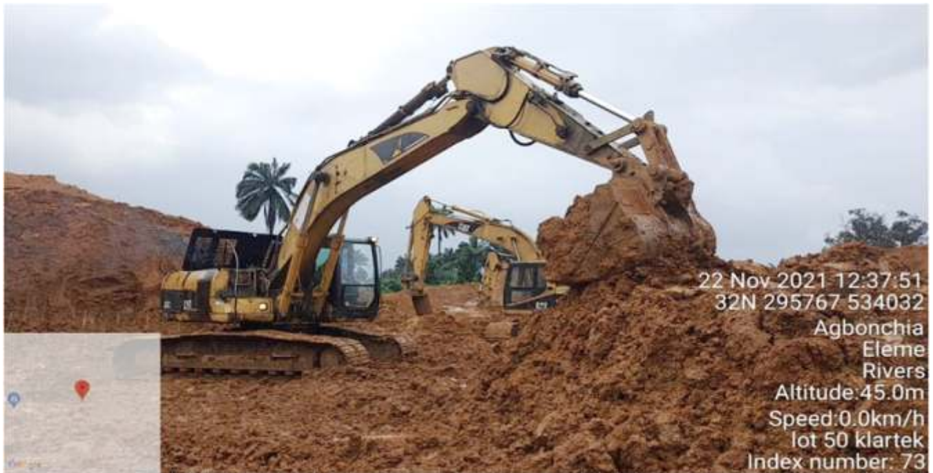
Plate 1.3: Serial transfer of treat soil for backfilling on-going at Lot 050 Okuluebu, Ogale , Eleme L.G.A. Remediation Contractor - KLARTEK NIG. LTD.
