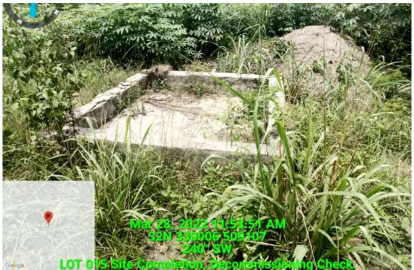
Plate 1.12: Yet to be decommissioned concrete base of the decontamination area at Lot 015 (Wiieborsi -Kpean, Khana L.G.A).
