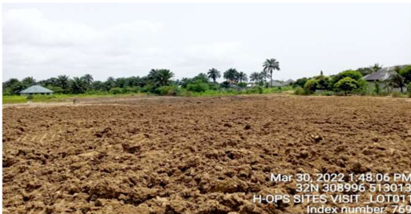
Plate 1.1: A panoramic view of Lot 011 at Debon, Bodo/Mogho, Gokana L.G.A. where final backfilling of excavated pits with the treated soil was recently concluded. (Contractor: MOSVINNY NIG. LTD).
