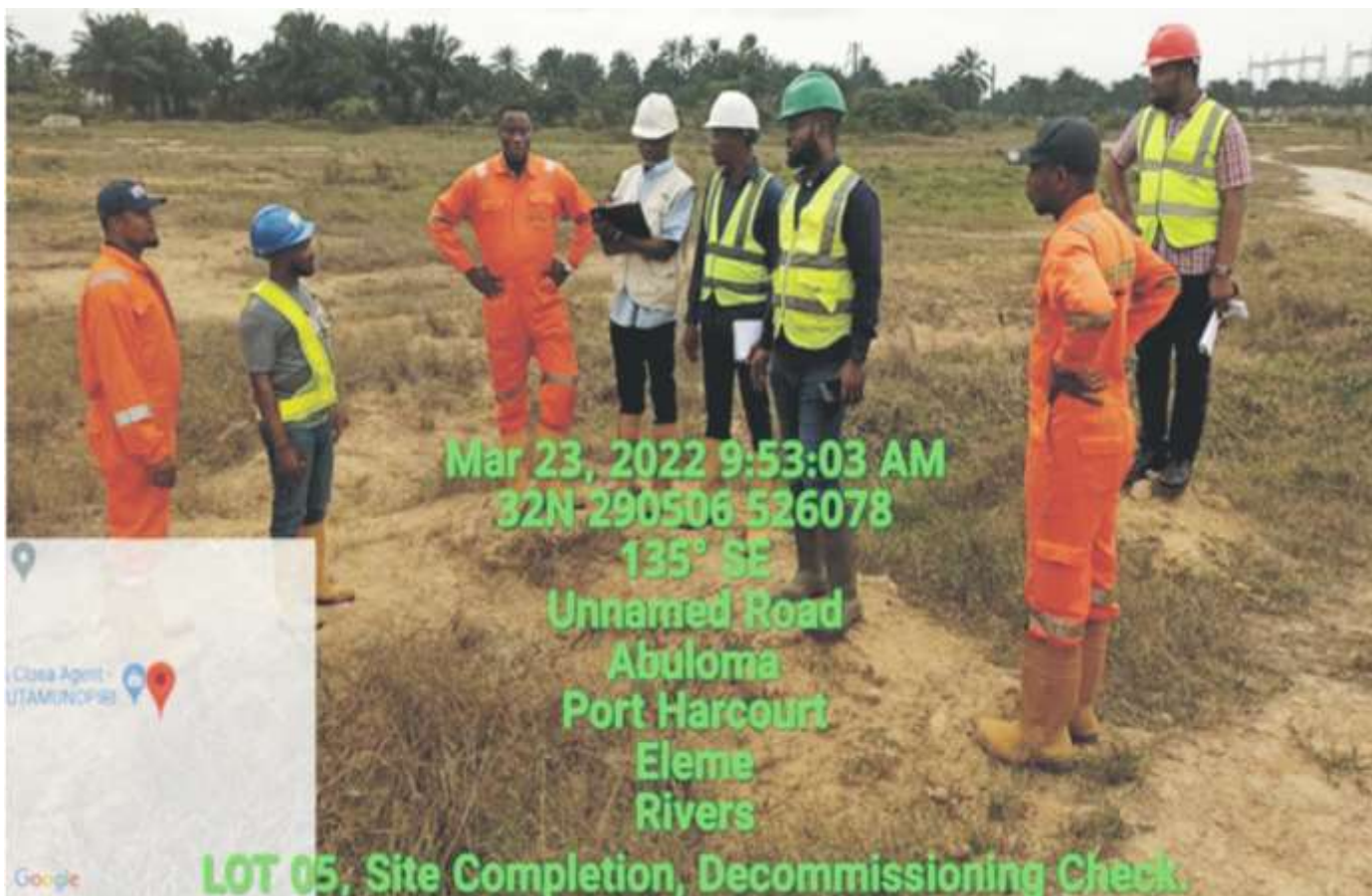
Plate 1.9: Team of Remediation Supervisors undertaking checks on levels of compliance with completion of remediation earthworks and decommissioning of site facilities at Lot 005 (Nkeleoken –Alode, Eleme L.G.A).
