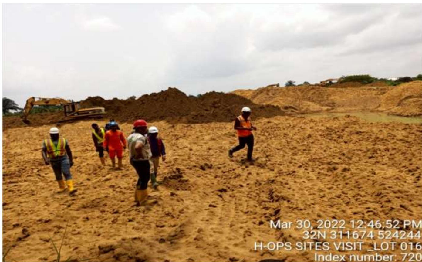
Plate 1.2: On-going backfilling of excavated pits with treated soil at Lot 016, Buemene Korokoro Well 005, Tai L.G.A. (Contractor: NEWLIN WEST AFRICA LTD)
