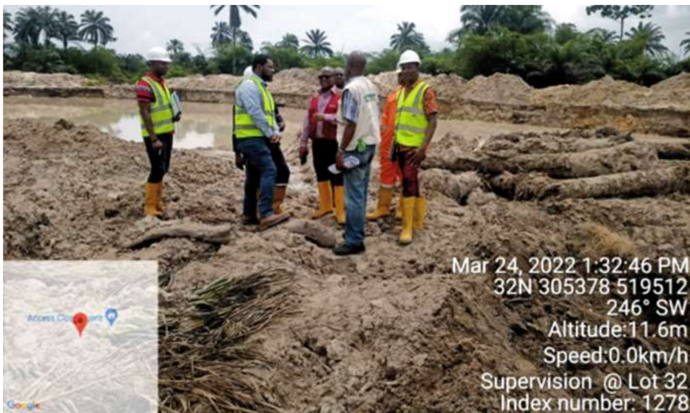
Plate 1.3: Excavation of impacted soil for treatment in progress at Lot 032 B-Dere/Gio, Gokana/Tai L.G.As. Remediation Contractor -MOSITO ENVIRONMENTAL LTD.
