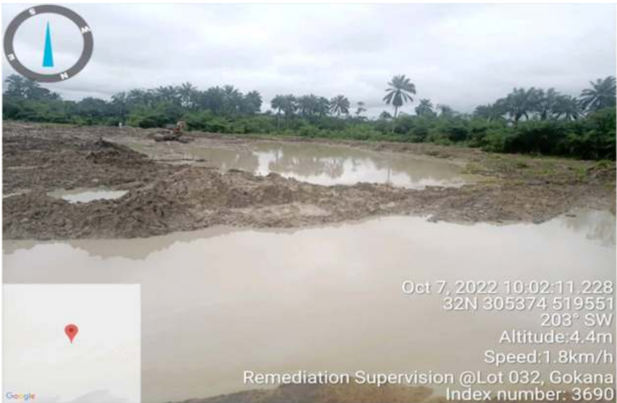
Plate 2.3: Overview of the Excavated Pit at Lot 032 -B. Dere/Gioin Gokana / Tai LGA.
