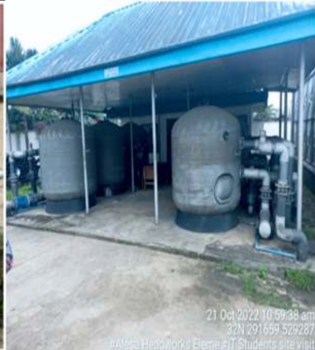
Plate 4.2b: Filtration system at Alesa Headworks
