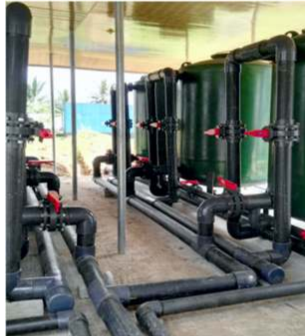
Plate 4.4b: Internal connection of pressure filters at Terabor station.
