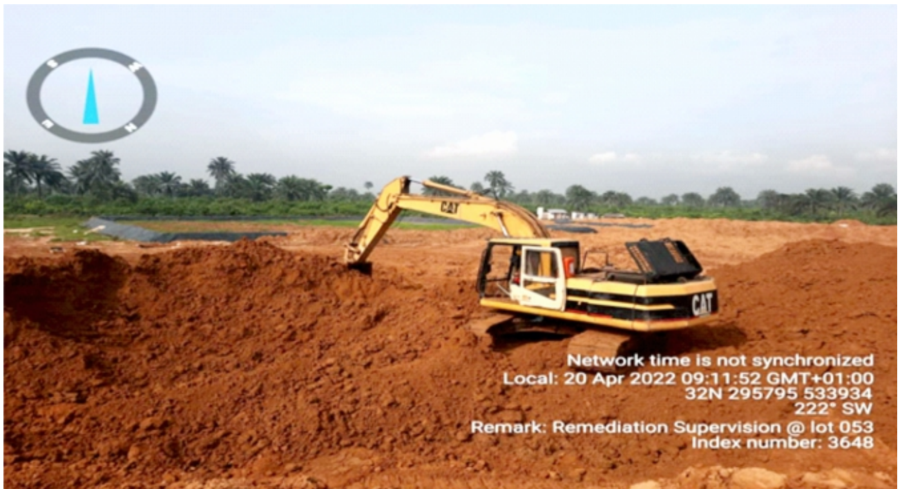
Plate 1.4: Transfer of Treated Soil from Storage Area to Excavated Pit for Backfilling at Lot 053 (Okuluebu Ajeokpori Well 3, Ogale, Eleme L.G.A) Remediation Contractor - ATLAS RAY AND SONS COY LTD.
