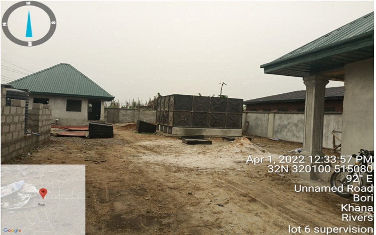
BOOSTER STATION AT A GLANCE AT BORI
