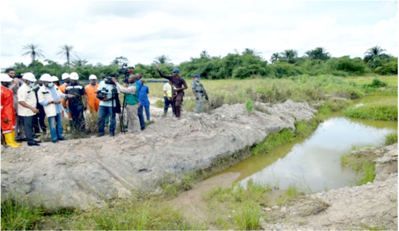
Plate 1.18: The Honourable Minister for Environment observing excavated pit partly backfilled during his visit to HYPREP Remediation site in B-Dere/Gio Gokana/Tai LGA.
