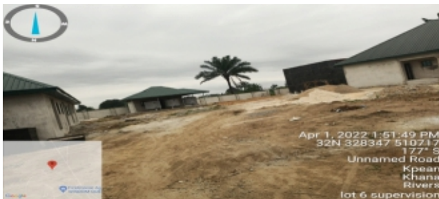
KPEAN HEADWORK AT A GLANCE
