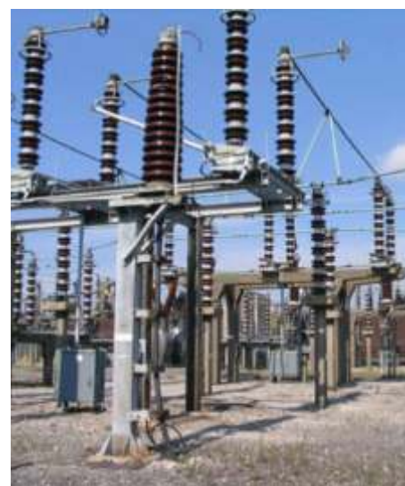
Power Sub Station
