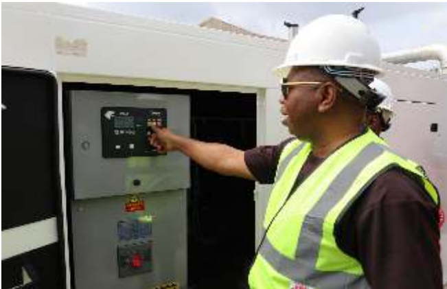
Dr. Giadom Turns on Switch of Generating Set to Power Project Office
