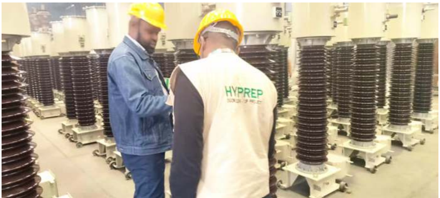
Factory Acceptance Test (FAT) for the offshore Components of the Ogoni Power Project
