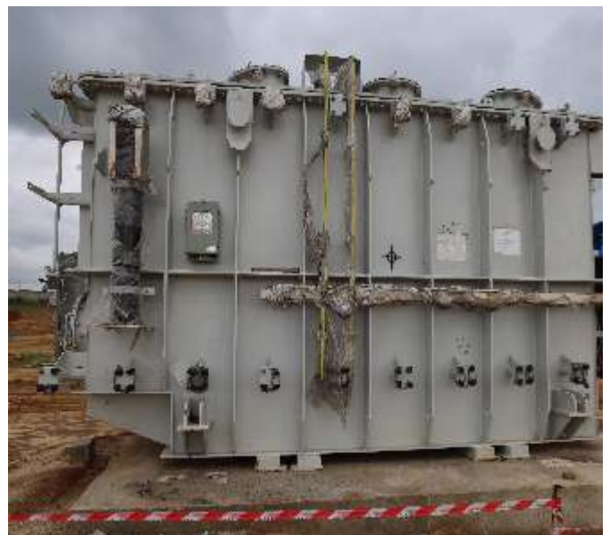
60MVA Power Transformer
