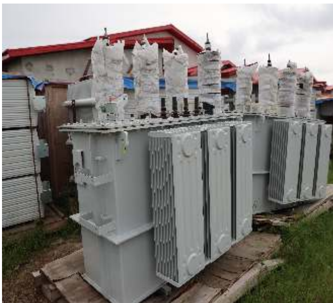
Transformer Cooling System
