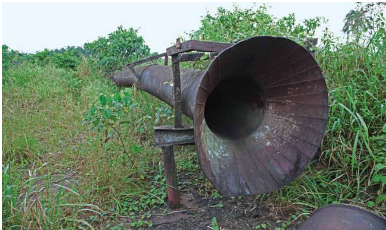
Flare arrangements at disused flow station
