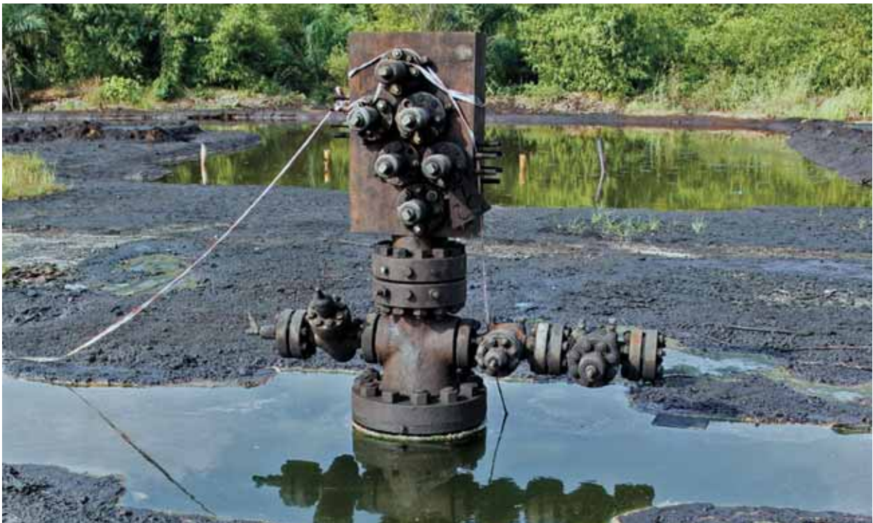
Easily accessible disused wellhead (Bomu 27, Gokana LGA)
