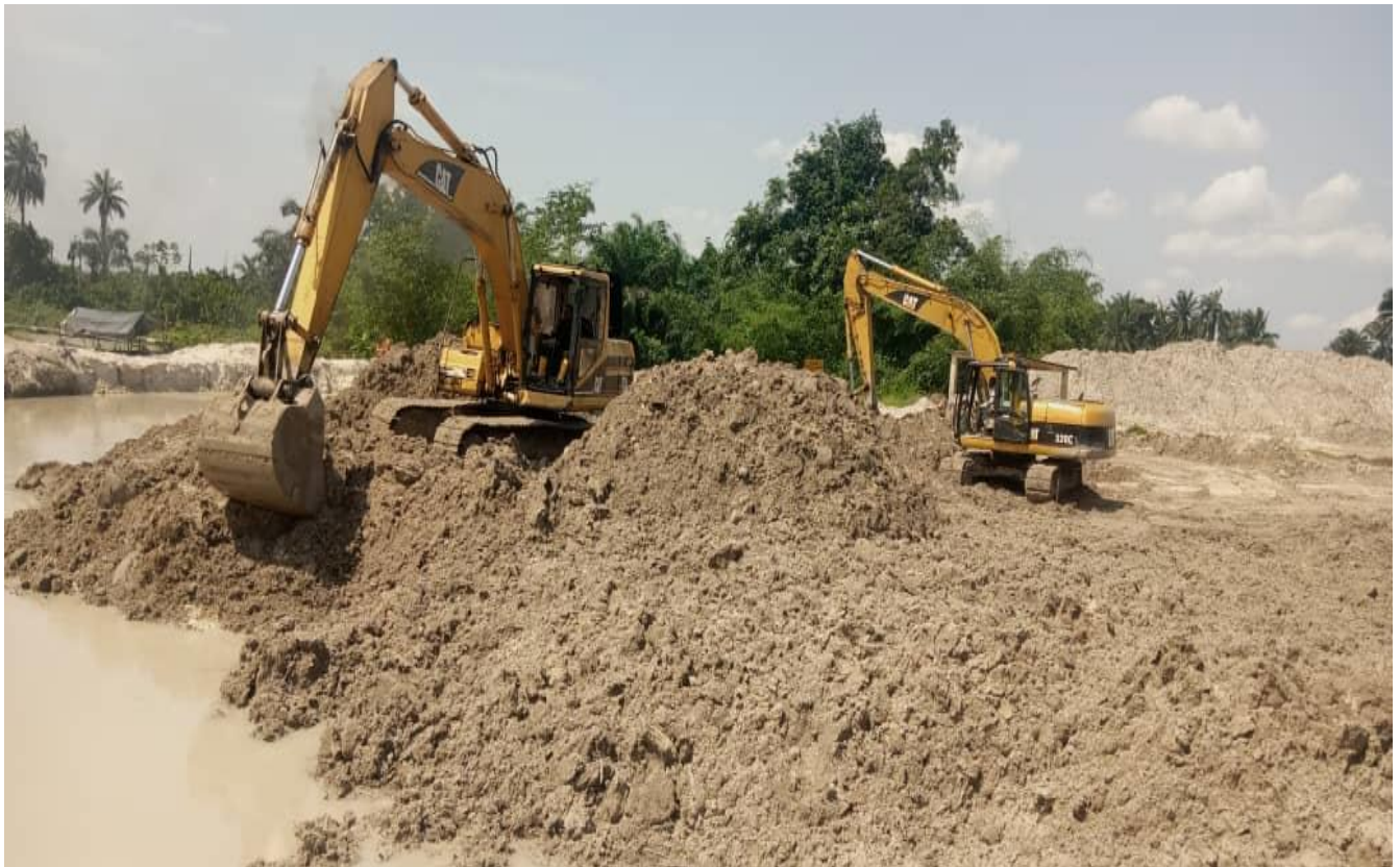
Plate 1: Backfilling of excavated pit with treated soil at Lot 009 (Saanako) in Mogho, Gokana L.G.A. (Contractor: Odun Environmental Ltd).
