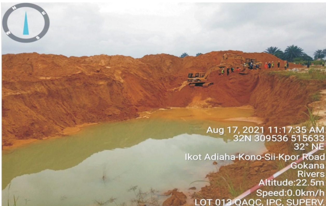
Plate 1.1: Ongoing mechanical excavation at Lot 013 (Nweekol Zorbuke) in K. Dere, Gokana L.G.A. (Contractor: CENTENNIAL DEVELOPMENT & INVESTMENTS LTD).
