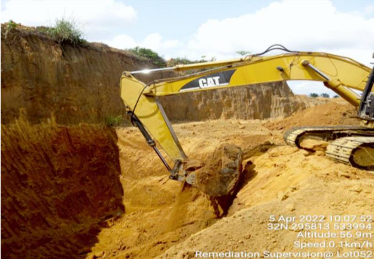
Plate 1.3: Excavation of impacted soil for treatment in progress at Lot 052 Okuluebu Ajeokpori Well 3, Ogale Eleme L.G.A. Remediation Contractor - MONTEGO UPSTREAM SERVICES LTD.
