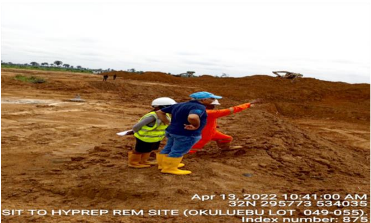
Plate 1.13: UNEP Representative and the Officer Overseeing HYPREP Operations Unit (Orange Coverall) examining Remediation Works been carried out in Okuluebu Ogale during one of his routine leadership commitment supervisory site visits on 13th April, 2022.
