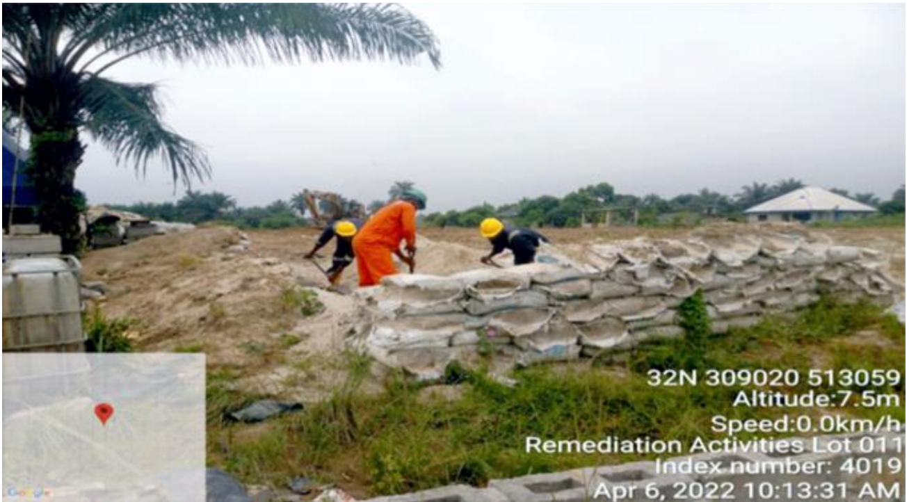
Plate 1.2: Decommissioning of Engineered Biocell after the Completion of Remediation Works at Lot 011 Debon Mogho/Bodo, Gokana LGA (Contractor: MOSVINNY NIG. LTD)
