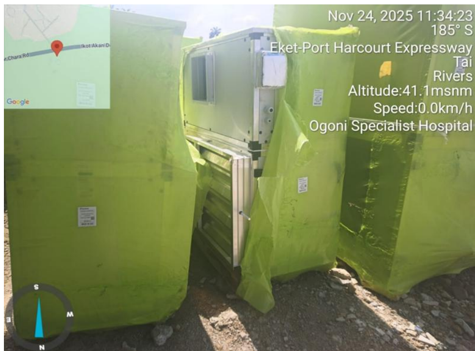
Air Handling Units (AHU)
