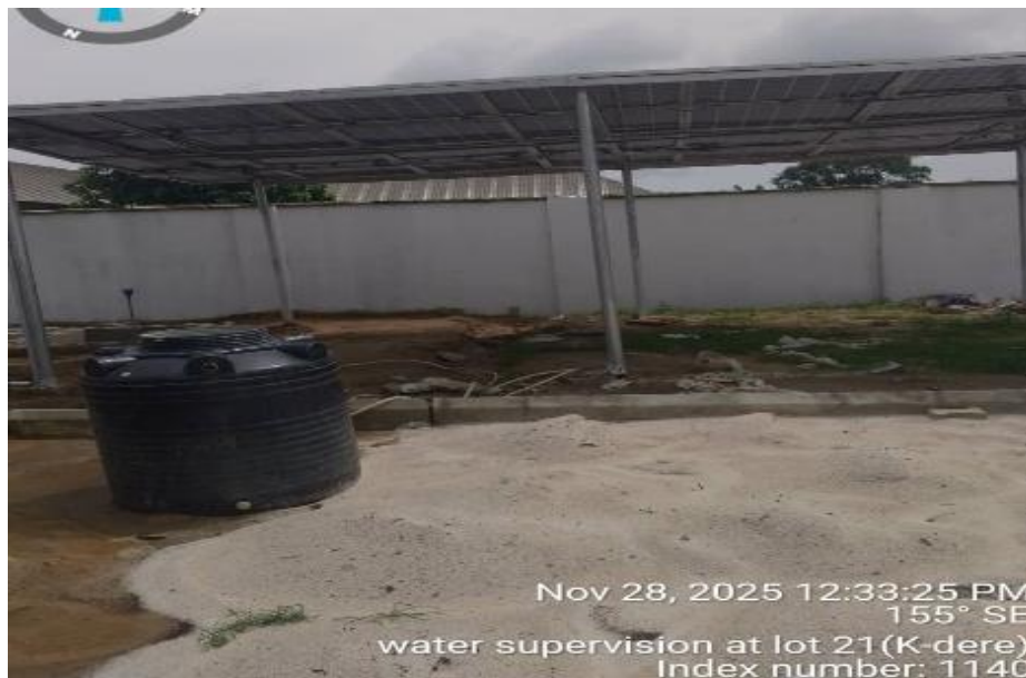
Solar installation at K-Dere site
