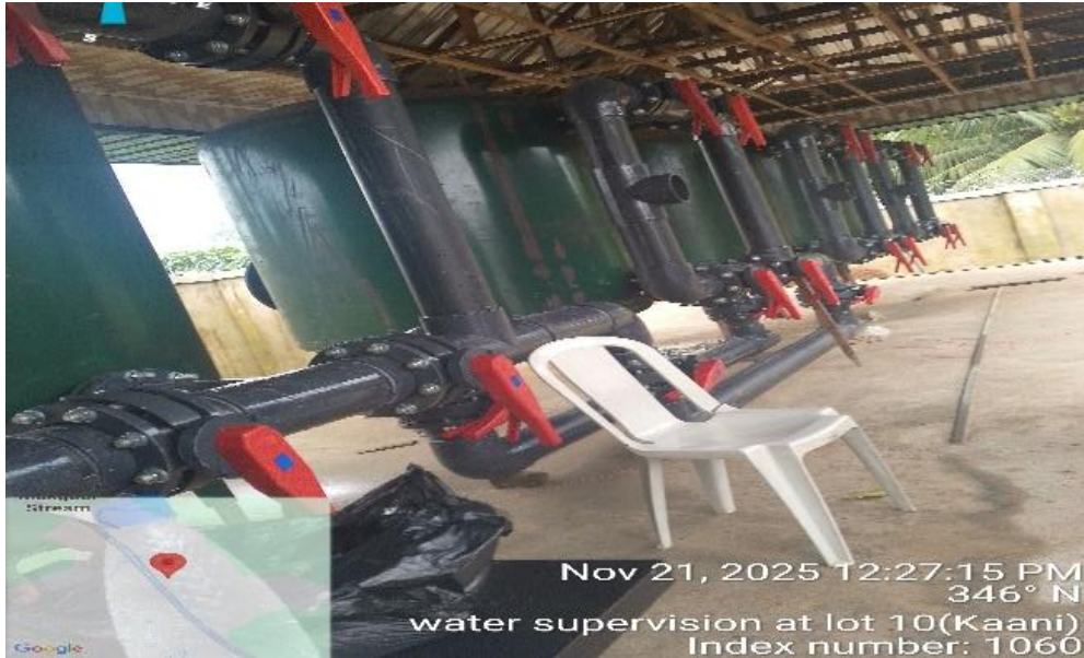
Ground tank at Bodo Station
