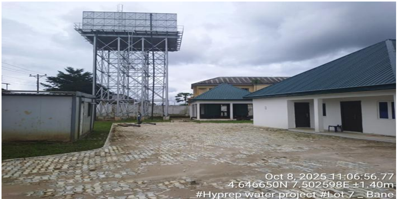
Bane Station getting set for commissioning
