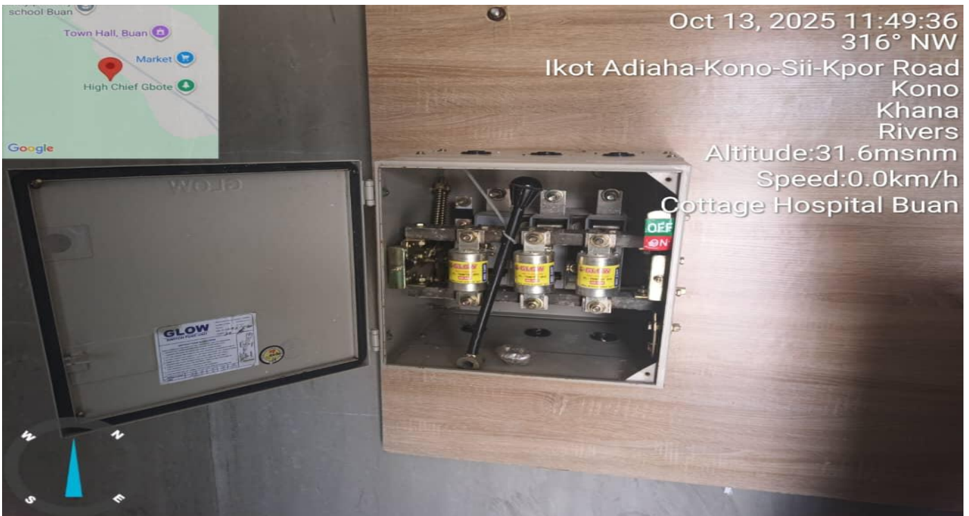
GEAR SWITCH BUS INSTALLED
