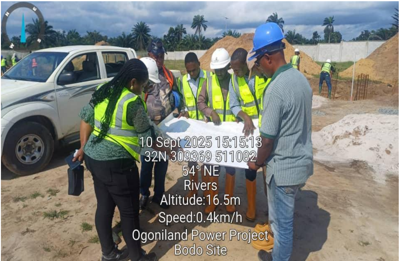
Figure1: HYPREP Staff, Consultant and Contractor Look at the switchyard layout design at Bodo substation (Gokana LGA)
